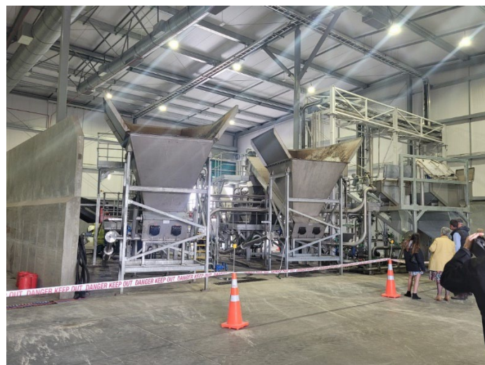
Figure 46: Sorting hoppers which receive and filter organic waste streams at Ecogas’ Reporoa plant.
