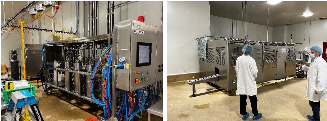
Figure 17 (left to right): CO 2 super critical extraction technology for extracting high value naturally occurring bioactives; FoodBowl Chief Executive, Grant Verry, shows the team a high pressure processing system, which can be used to non-thermally preserve food, extending shelf-life and preventing waste while maintaining the sensory and nutritional properties of the food product.
