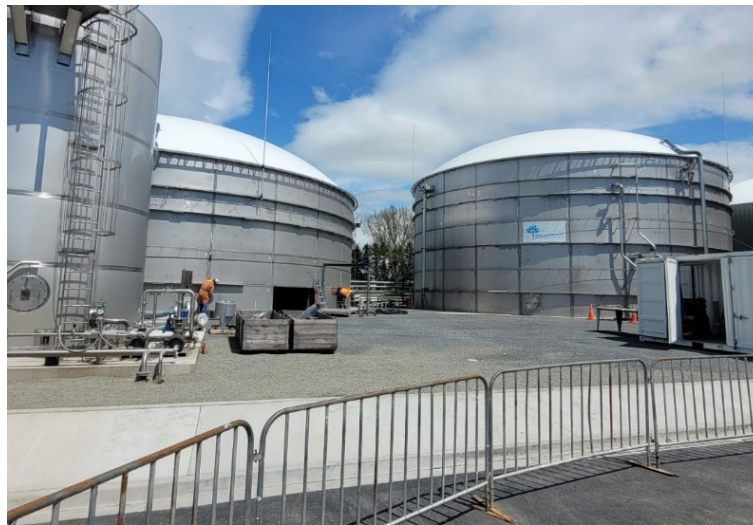
Figure 47: The digester tanks at Reporoa which hold up to 3.5 million litres of organic waste. Methane rises to the top of the tanks and are captured using a hose system.
